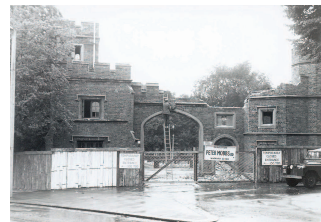
Demolition of the Lodge Gates in 1970, in line with the widening of Rickmansworth Road (old road alignment bottom left of photo)
