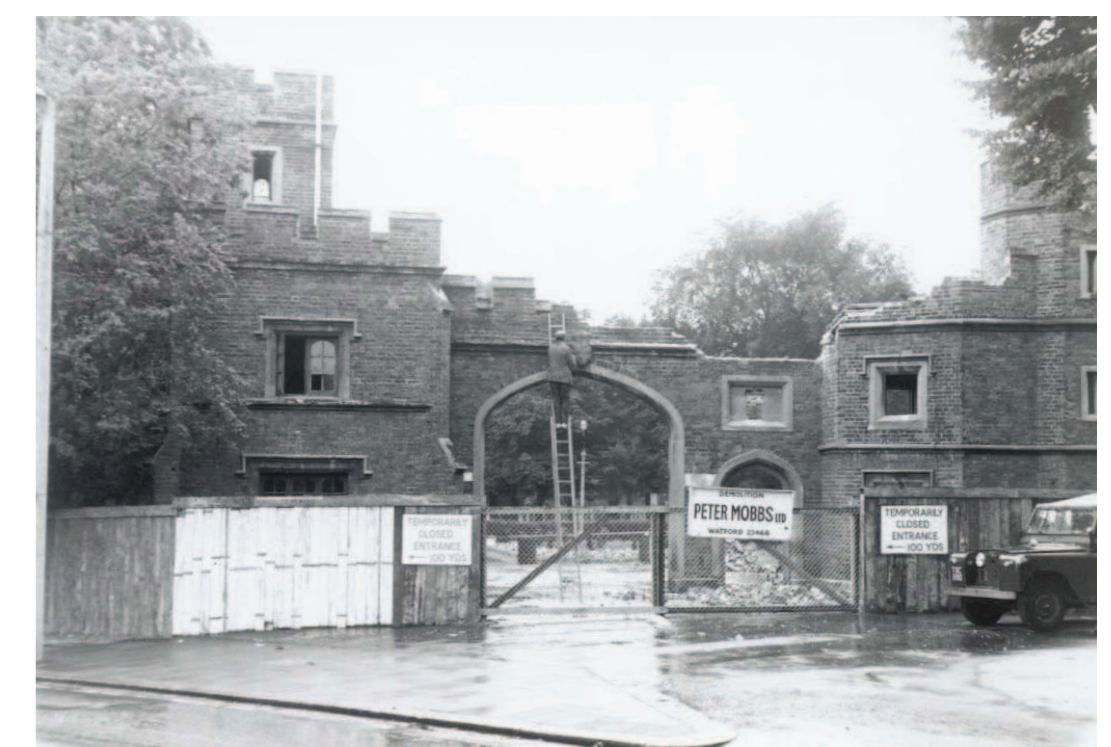
Demolition of the Lodge Gates in 1970, in line with the widening of Rickmansworth Road (old road alignment bottom left of photo)
